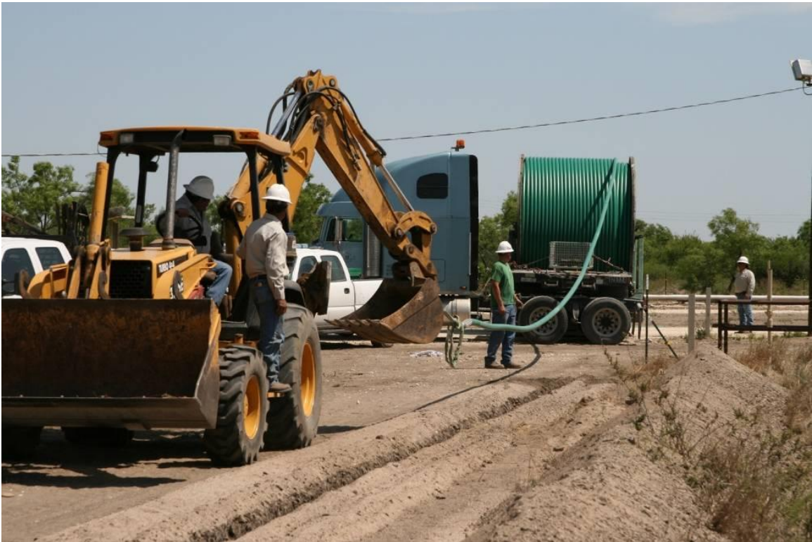
Figure 7-5 Spoolable Composite Pipe (SCP) - Unreeing Pipe for Placement in Pipeline Trench. (Photo used courtesy of Fiberspar LinePipe Canada Ltd)
