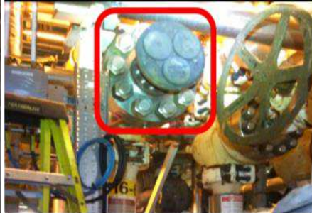
Upper diverter valve following event
