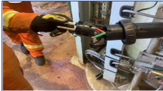
Fig 2: Loose Ground on Temp Power Cord (Internal Inspection)
