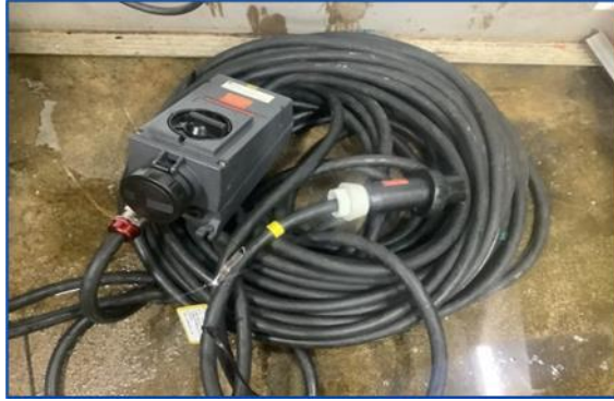
Fig 1: Temporary Cable with disconnected ground (green)
