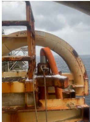
Fig. 1. Potable Water Hose Showing the Kink
